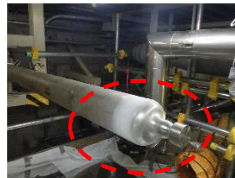
After isolation (inlet pipe for the intermediate heat exchanger)
