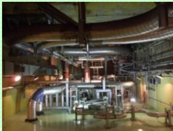
Main steam piping
