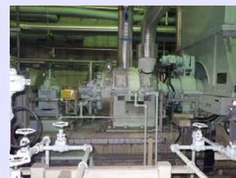
Main feedwater pump
