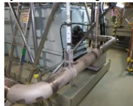
Preheating/warming equipment (after dismantling)
