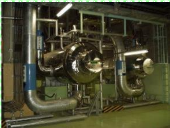
Nos. 3 & 4 feedwater heaters
