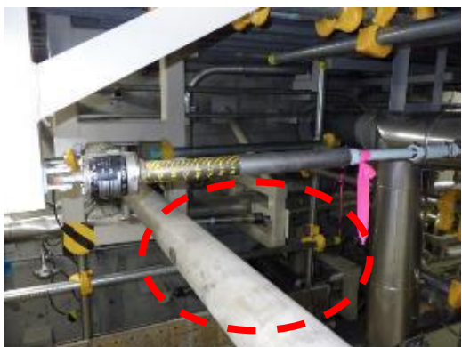
Before isolation (inlet pipe for the intermediate heat exchanger)
