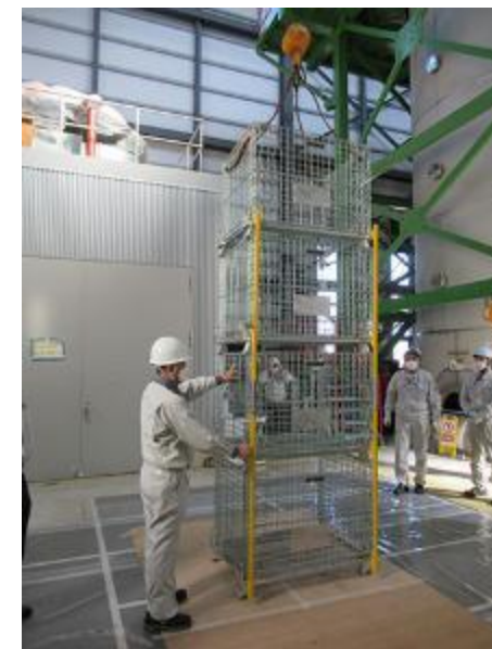
Prototype installation test (four layers)
