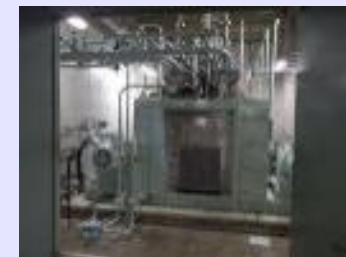
Oil tank (high-pressure oil unit)
