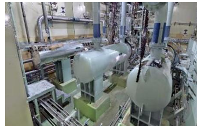
Data for MR obtained by laser scanner (Fugen sodium cleaning system)
