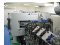
Radiopharmaceutical manufacturing facility
