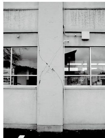
A pillar of a school building cracked by the Niigata-Chuetsu Earthquake. (Ojiya City, Niigata Prefecture)
