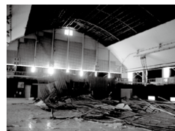
A Ceiling of a gymnasium collapsed partially due to the Niigata-Chuetsu Earthquake (Unuma City, Niigata Prefecture)
